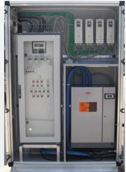
Front section of the technical compartment
