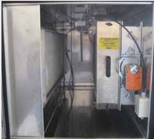
Return section with recovery coils
