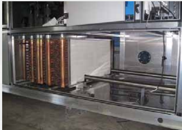
Humidification chamber and treatment coils with upper technical compartment for housing valves and recovery system circuit
